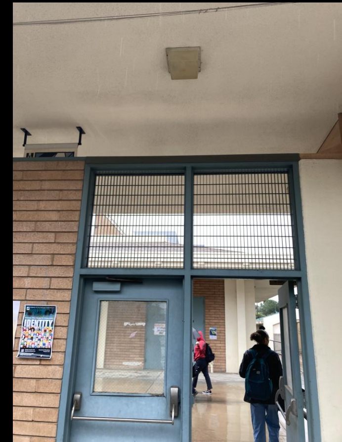
3. Grating above doors that access the Art courtyard in the middle of bldgs. 24, 25, 26, 27
